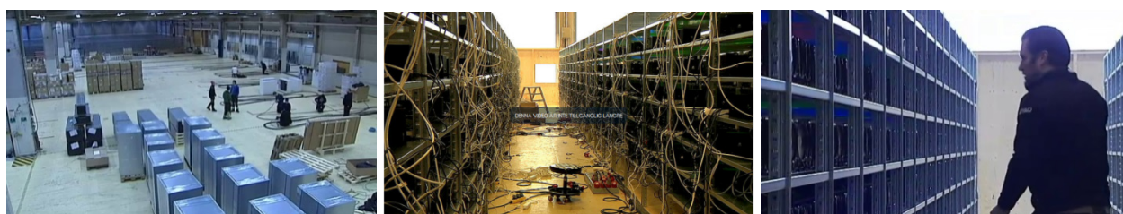
Figure 4: The KnC Miner Data Center in Sweden
